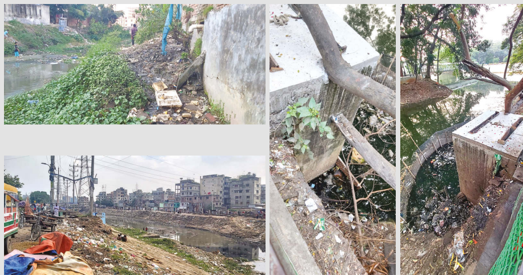
Figure 7.5: Dumped solid waste and sedimented Ramchandrapur Canal near Basila area (Upper right), Dumped solid waste in the old Buriganga riverside even after the dredging works (Lower right), damaged and broken culvert in Dhanmondi 32 (Left side)
